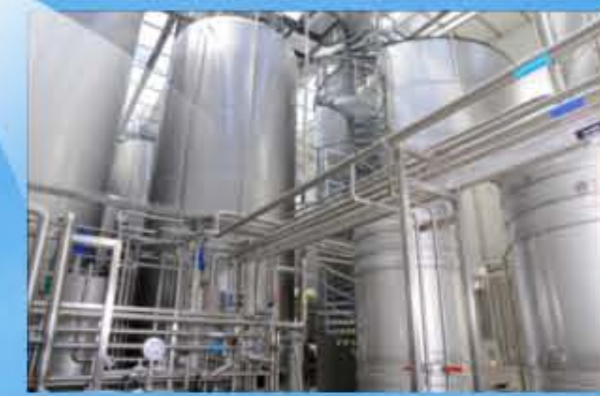
Stainless Steel Casting for Process Equipments
